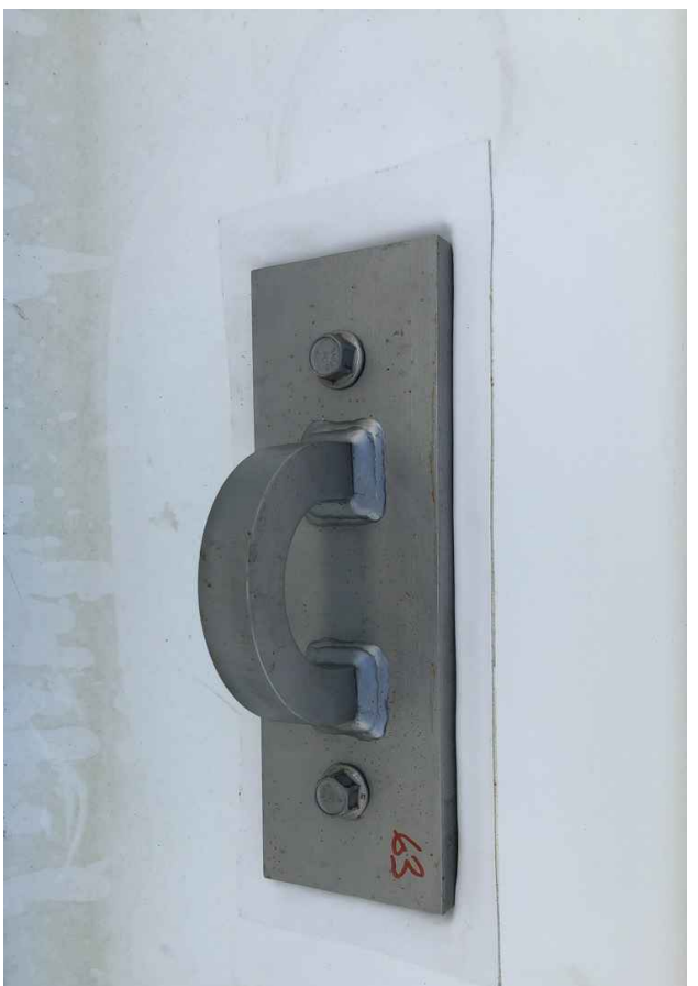
South Hampton - Roof Anchor #63 - pretest.
