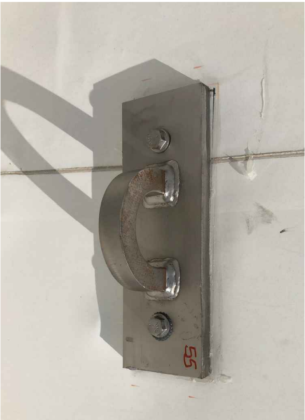
South Hampton - Roof Anchor #55 - pretest.
