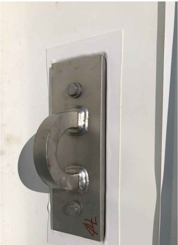
South Hampton - Roof Anchor #70 - pretest.
