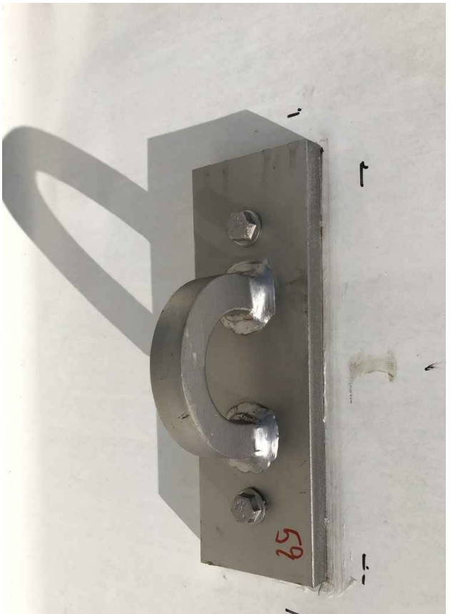
South Hampton - Roof Anchor #59 - pretest.
