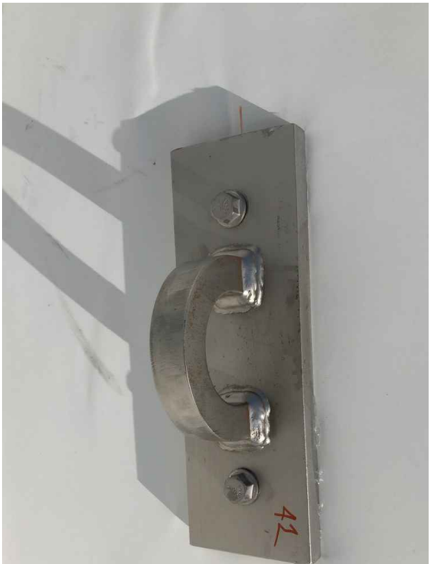
South Hampton - Roof Anchor #42 - pretest.
