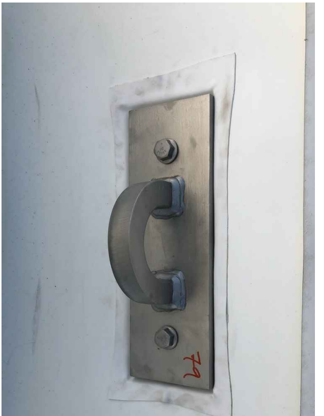
South Hampton - Roof Anchor #79 - pretest.
