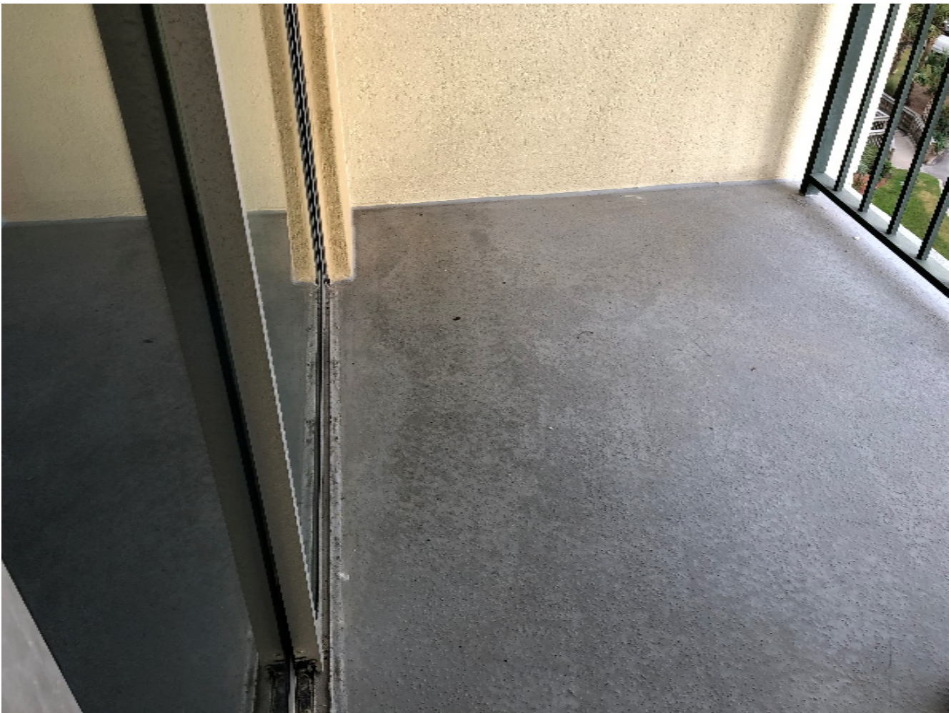
Figure #1 – Ponding due to Negative Slope
